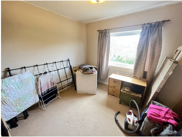
Rear window, radiator
